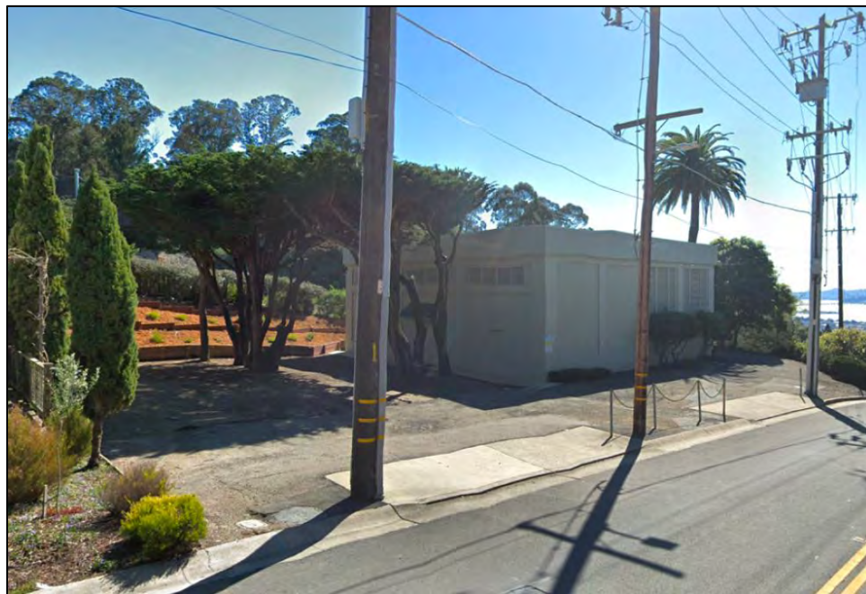
Figure 17: PG&E Substation (Source: Alternatives Analysis).
